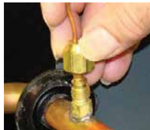
B. Screw flare nut on TXV equalization tube on to the Schrader valve stem.
